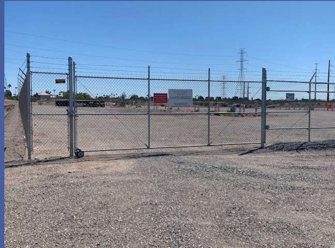
Battery Storage Site
