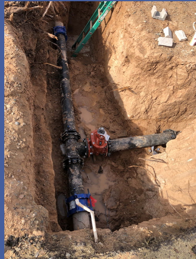
New Cut-In Tee/Valve Assembly
